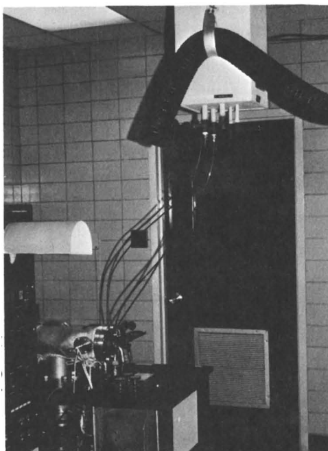
Figure 2. Service drops in instrumental laboratory. (a) Gas and electrical supply for differential thermal analysis and (b) cooling water and electrical connections to a mass spectrometer.
