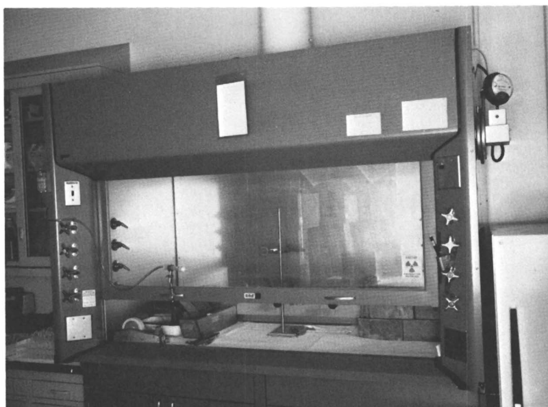
Figure 7. Chemical fume hood
